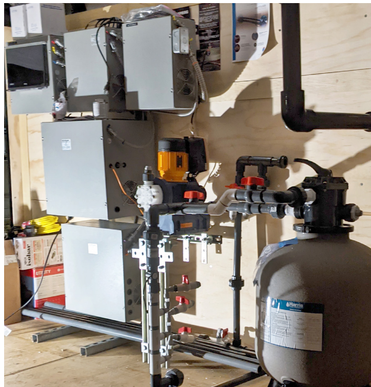
SafeGuard™ H2O trailer-mounted arsenic removal demonstration system installed at Isleton Well #3A.
